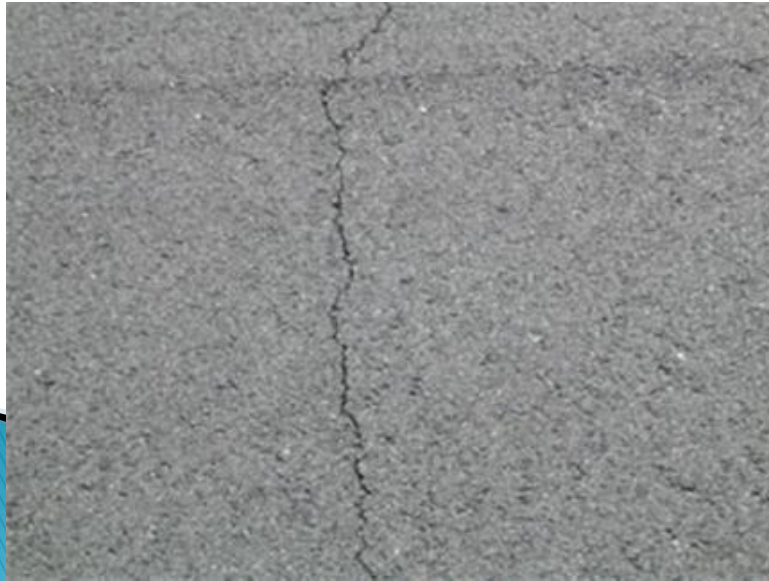
Plate 3: Transverse crack (Low temperature cracking)
