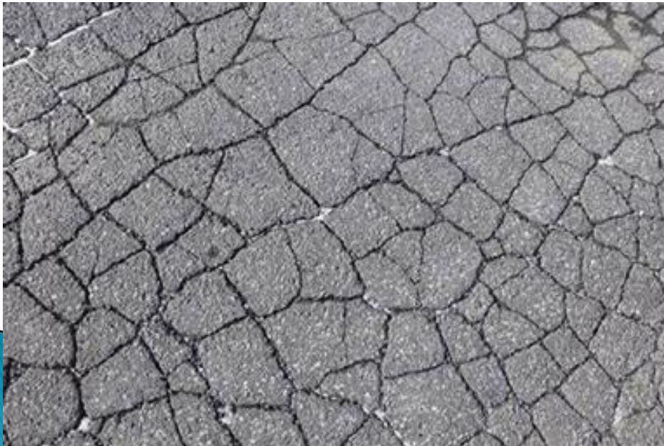
Plate 2: A typical pavement with fatigue cracking
