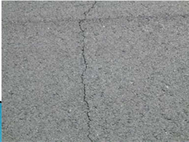
Plate 4: Transverse crack (Low temperature cracking)
