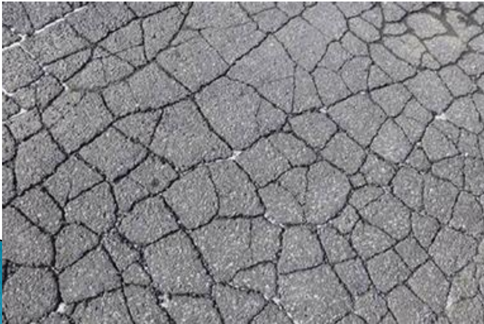
Plate 3: A typical pavement with fatigue cracking
