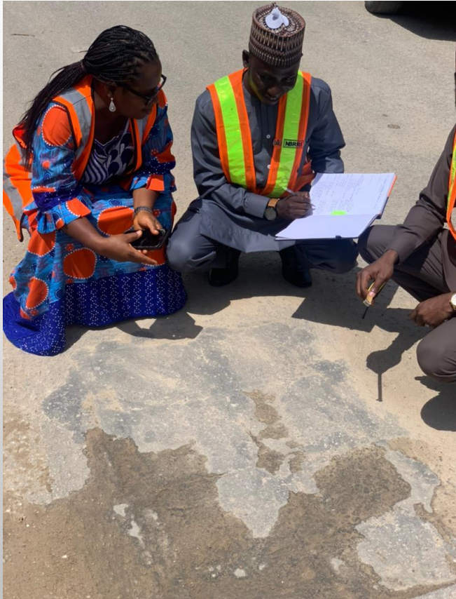
Patched surface during wet season
